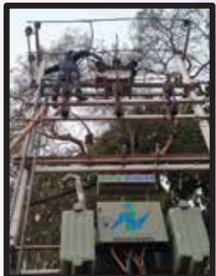
Gas releasing and tightness checking of jumper at metering unit of Aditya Vision near Planetarium.
