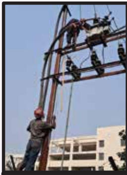
Flat earthing of cable and metering unit at state hanger.
