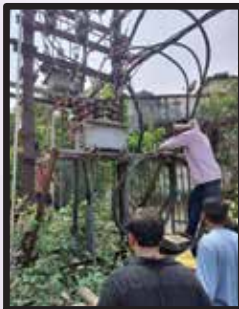
Placing PVC sheet between cable at Planetarium in 11 KV Gardiner Road feeder and PG 2 feeder.
