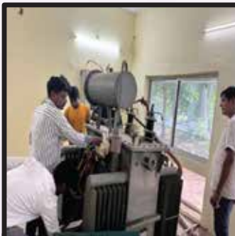
Maintenance in Raj Bhawan DTR.
